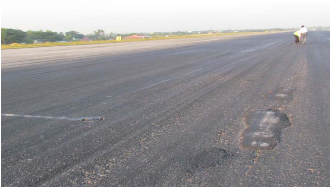
Figure (5) Scrape marks on the runway
